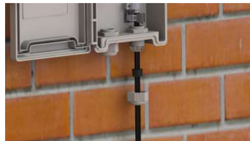
Fig. 6 Cable passed through the parts of the input port.
